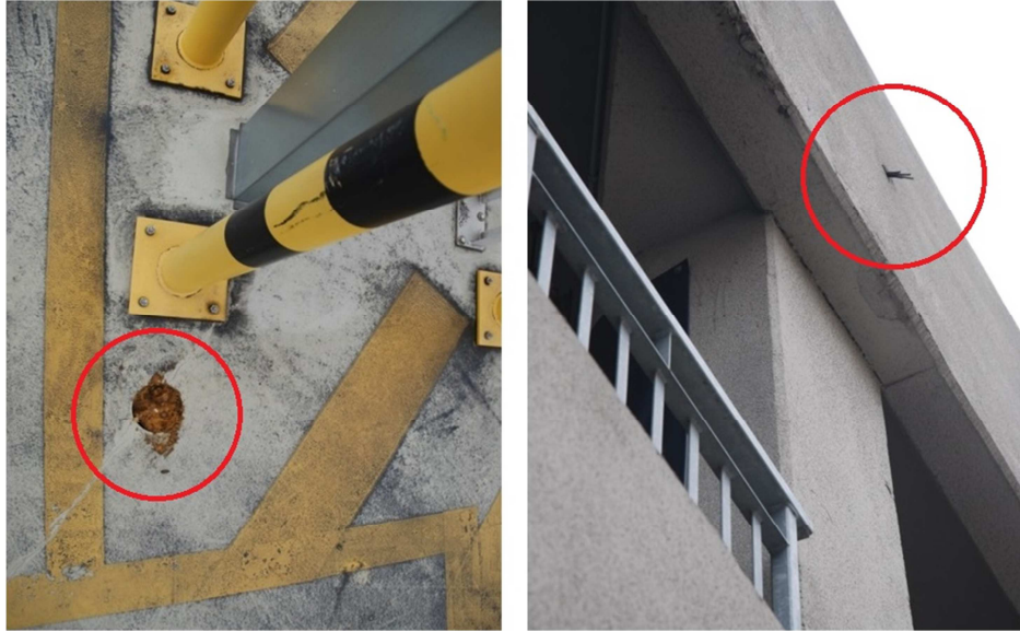
Figure 2. The intersection of the strand in the borehole (left picture) and its launch from the structure (right picture).
