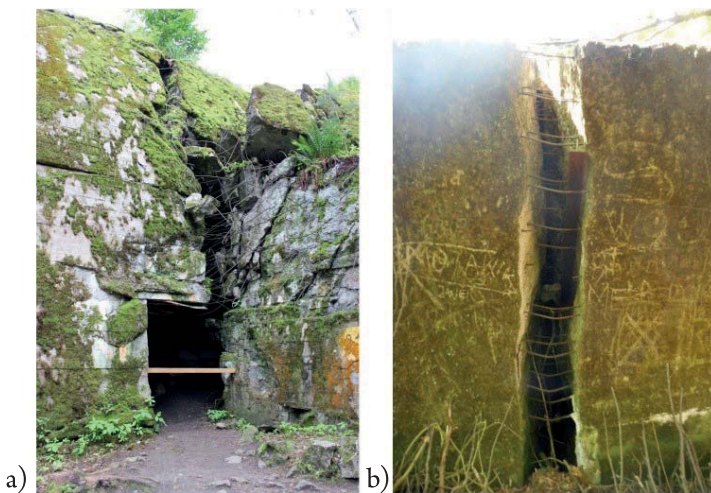
Fig. 14. View of the importance of reinforcement in ensuring ductility and compactness of concrete structures (own photos)
